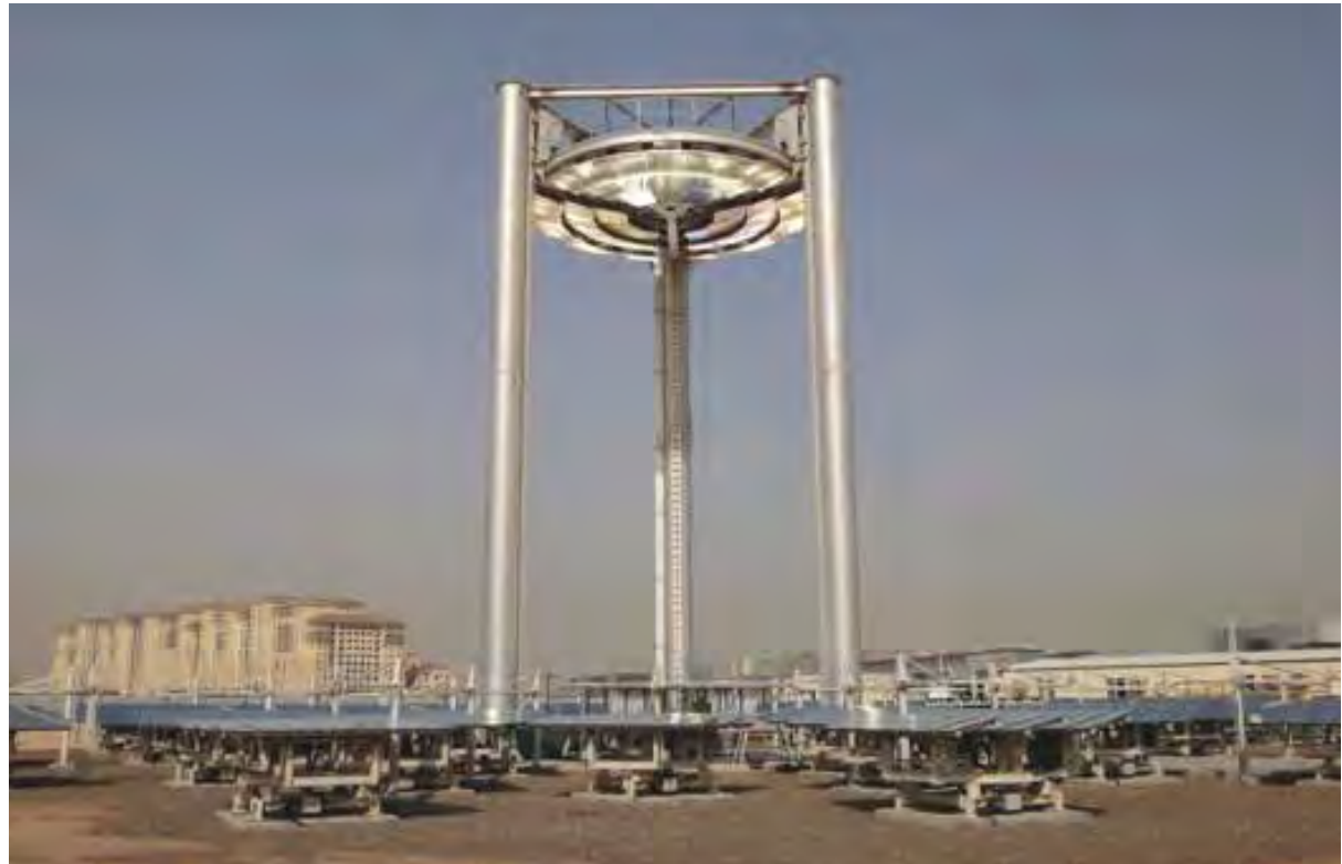
Beam-down point-focus CSP heliostat array at Masdar
