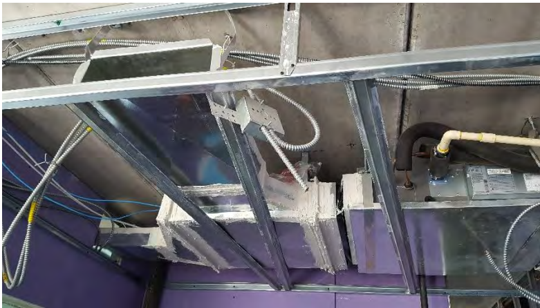
Ducted Ceiling Units
