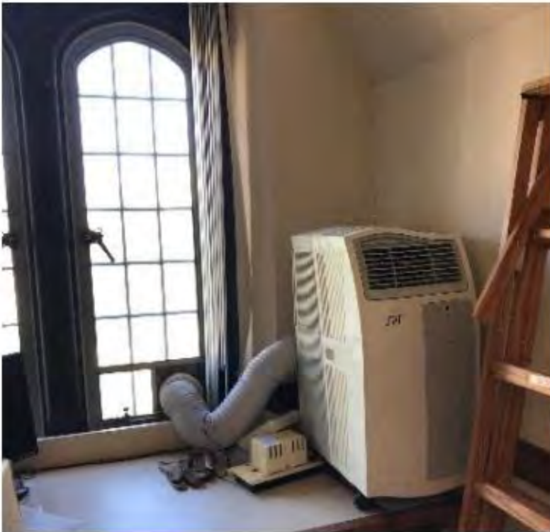
EXAMPLE OF LOCALIZED A/C UNIT LOCATED IN ROOM 403
