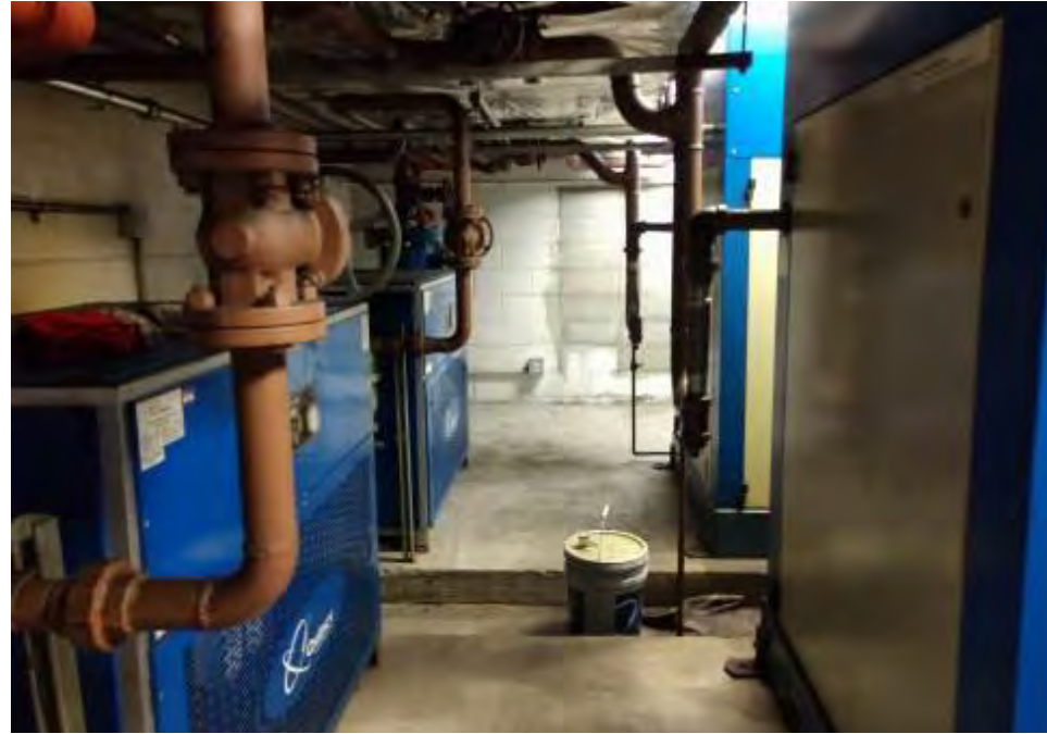
Compressor Room at DSNY District 4/4A/7 Garage
