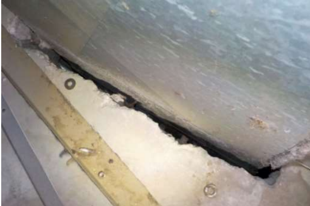
Air Gaps in Monitor Floor
