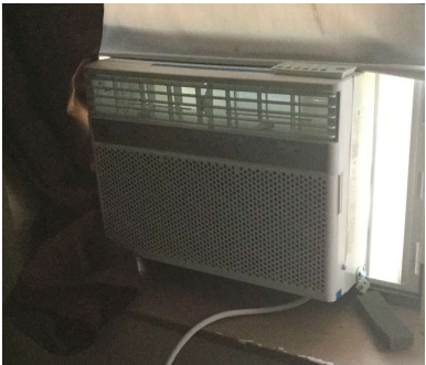
Window AC units
