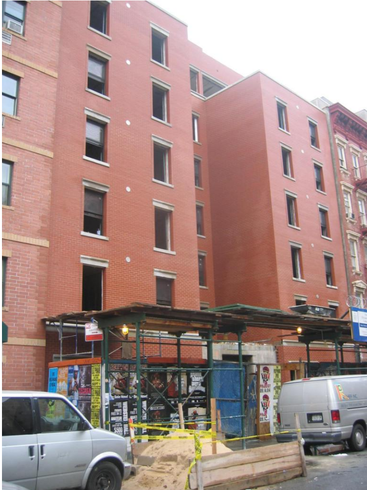
Passive House new multifamily in Brooklyn, NY – Photo Credit: Chris Benedict, RA
