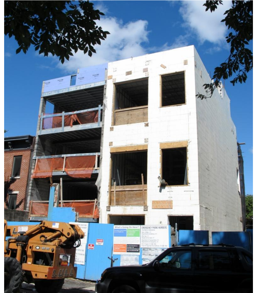
Three-unit, spec condo being built to Passive House standards in Brooklyn, NY – Photo Credit: A Wilson
