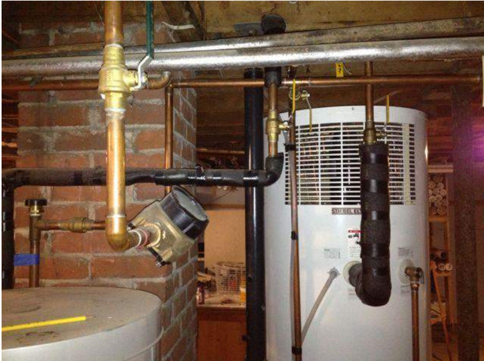
Hot Water Metering- flow meter on cold inlet
