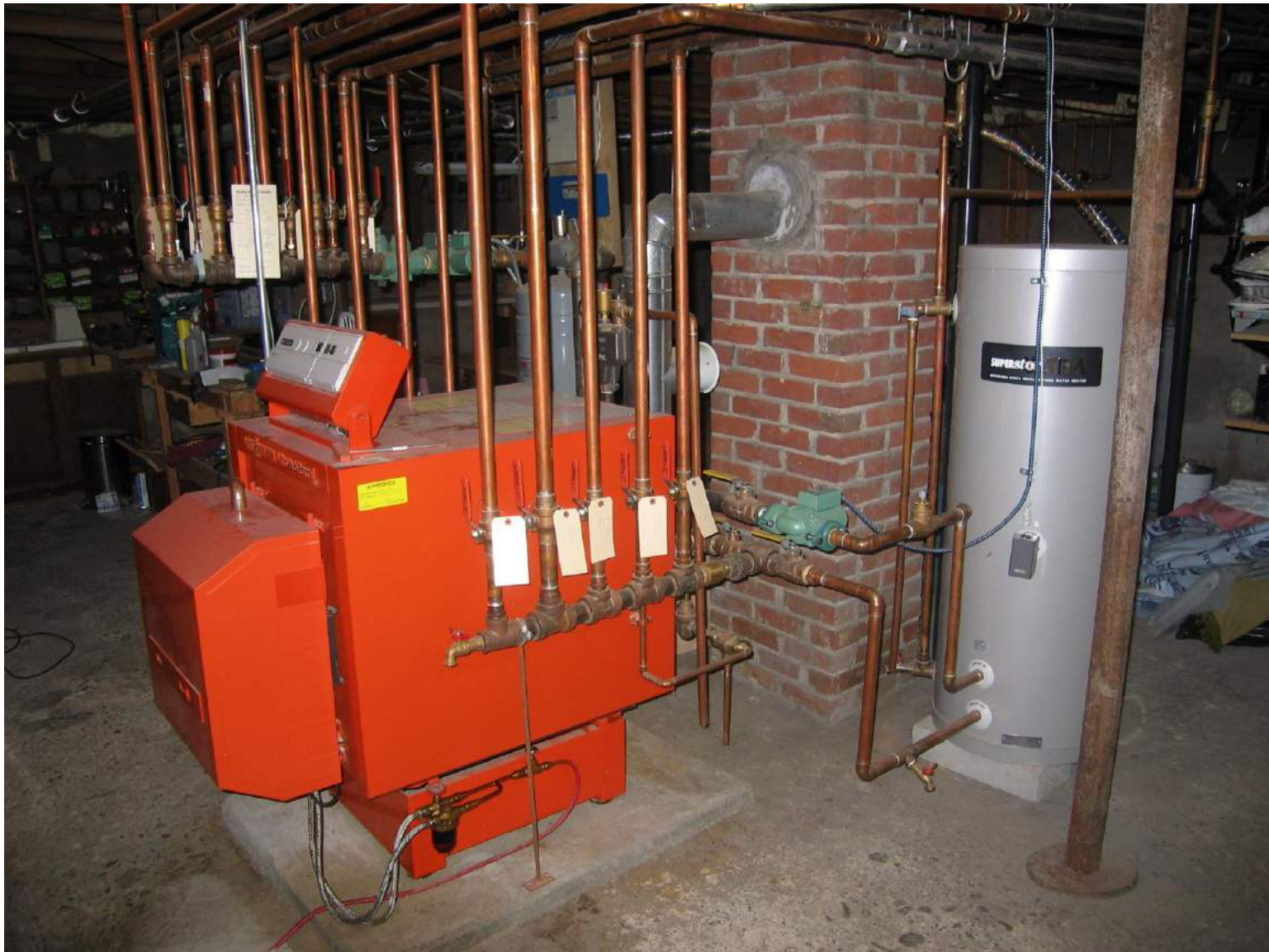
New boiler in 2000 and indirect tank for hot water in 2002
