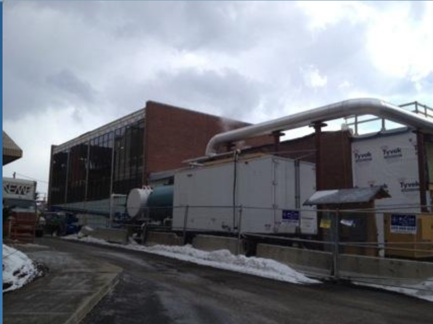
Montpelier, Vermont's district heat plant
