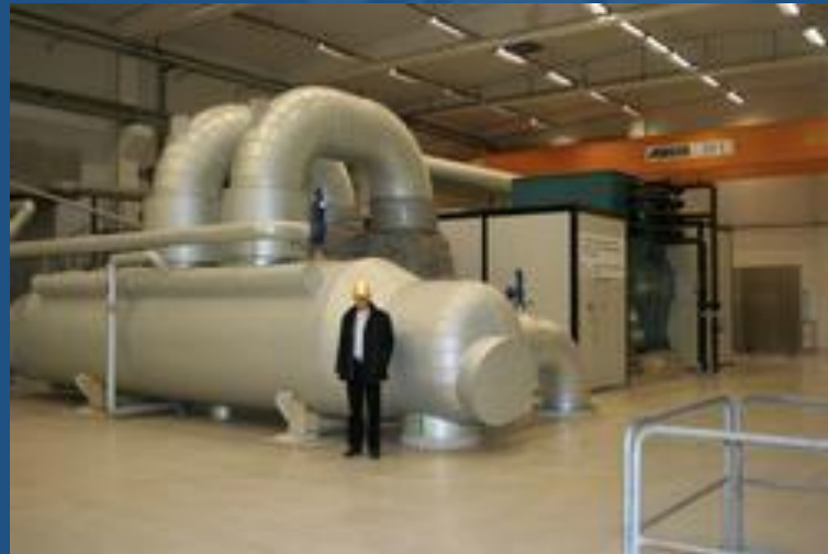
This CHP plant in Växjö, Sweden provides 29,000 customers with electricity and over 6,500 with heat.
